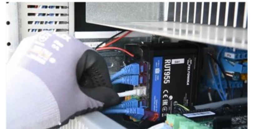
The Delta Electronics service connection is maintained through the integrated RUT955 router's wireless modem and a dedicated SIM card.
